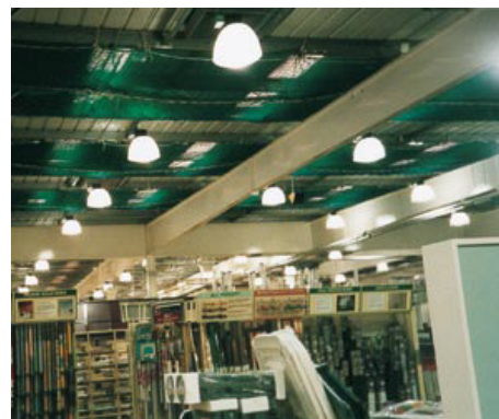
Safety netting protecting rooflights
