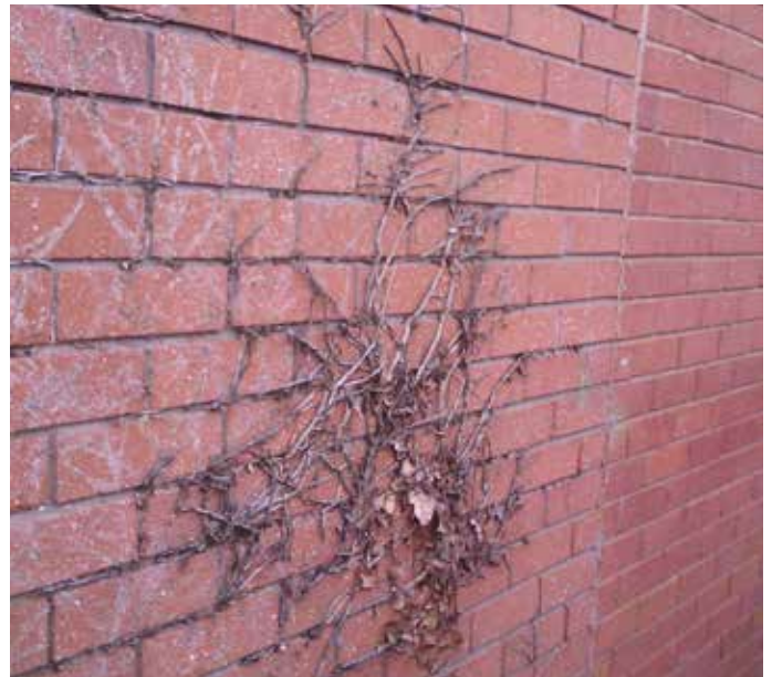
Figure 10: Plant growth and mould, indicating wet substrate
