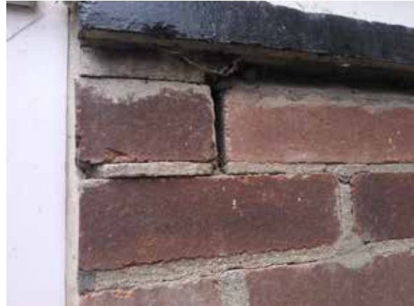
Figure 12: Cracked and missing
