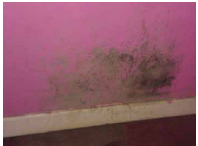
Figure 53: Damp behind a bed, removed for inspection
