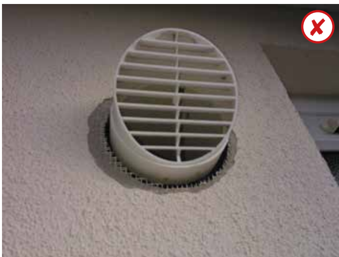
Figure 34: Unsealed extract fan in a bungalow
