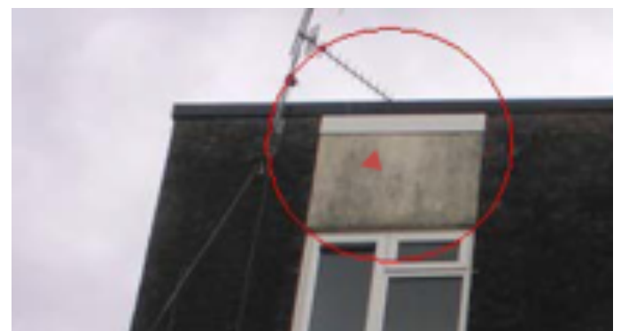
Figure 6: mould on saturated render panels
