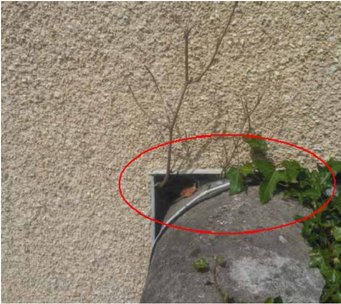
Figure 48: Plant growth allowed by poor detailing
