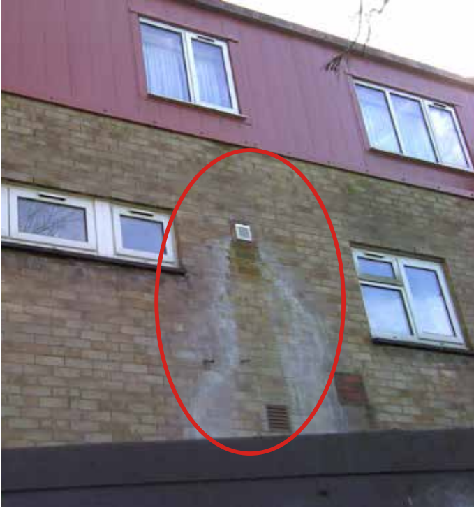
Figure 7: Water dripping from extract fan cover and staining the walls
