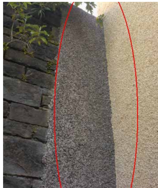
Figure 47: Cold bridge exacerbated by placement of insulation around an obstruction
