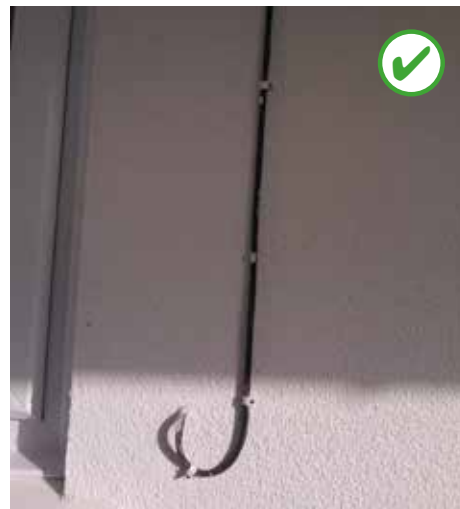
Figure 39 – cable clipped (good practice)
