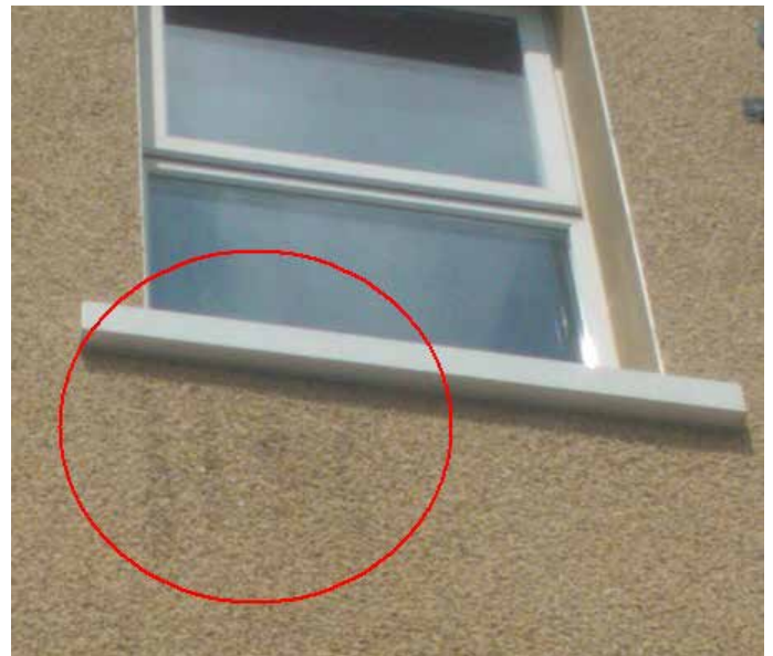
Figure 46: Incorrect finish of sill
