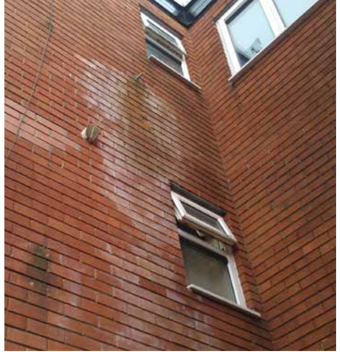
Figure 8: Leaking overflow pipe staining the brickwork
