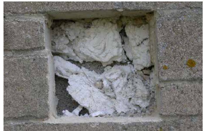
Figure 4: Example of saturated insulation
