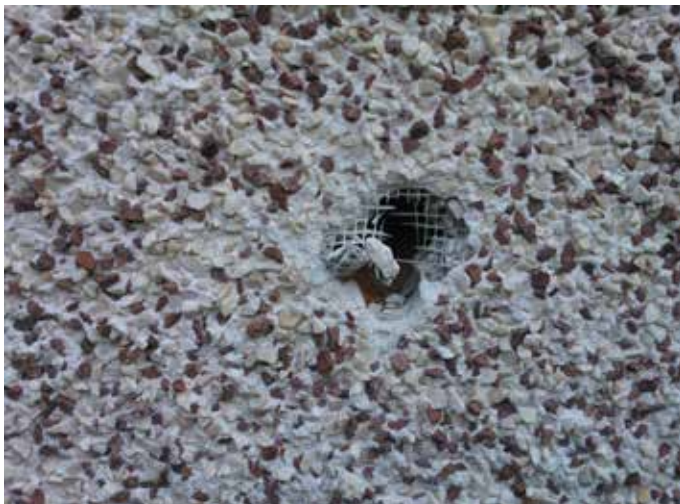
Figure 40: hole in a wall (from scaffolding used during construction)
