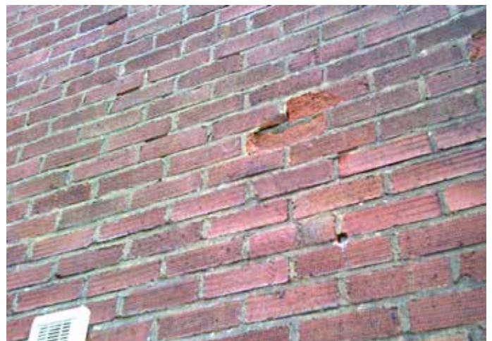
Figure 16: Missing brick faces
