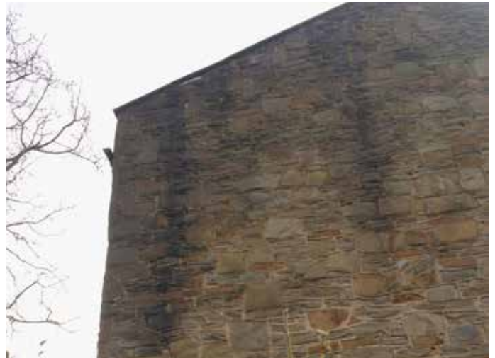
Figure 14: Staining from roof water run off
