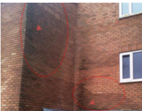
Figure 5: mould on saturated brickwork
