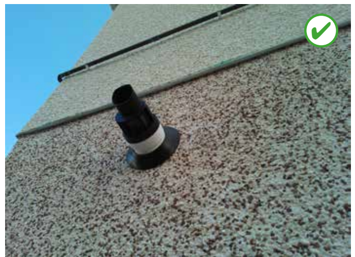
Figure 37: sealed penetration (good practice)
