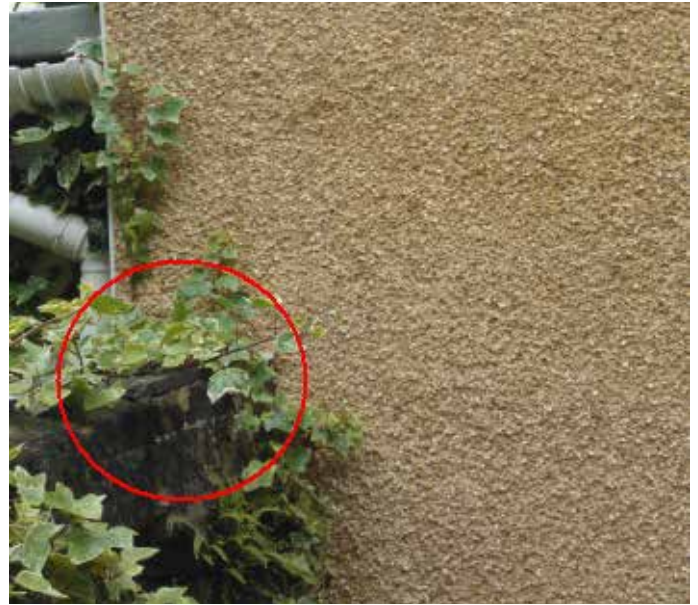
Figure 49: Close proximity of plant requiring pruning
