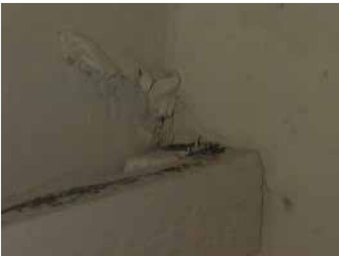
Figure 52: Damp in the wardrobe
