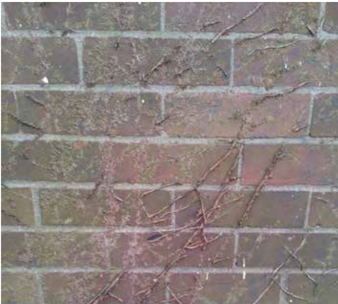
Figure 9: Plant growth attached to walls
