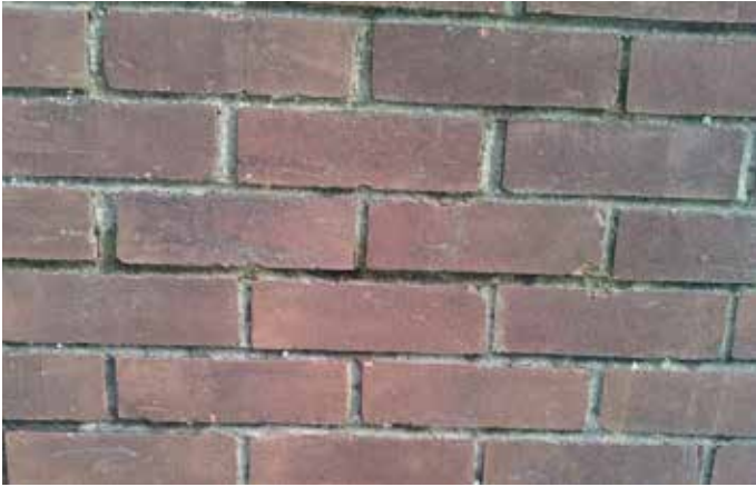
Figure 11: Erosion of mortar by weather
