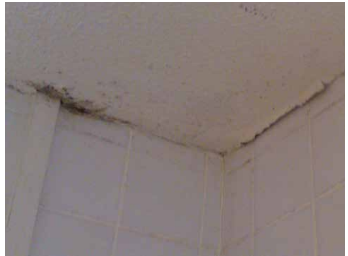
Figure 51: Damp in the bathroom
