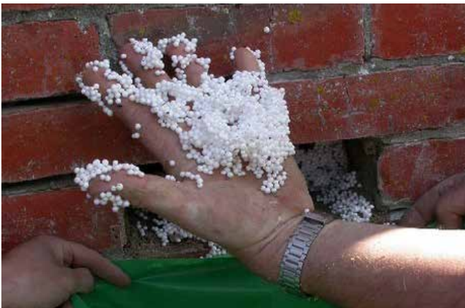
Figure 3: Example of saturated insulation
