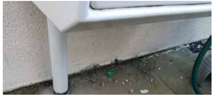
Figure 42: Penetrating damp potential in external wall finish
