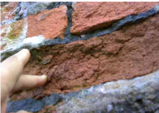
Figure 15: Significant brick face loss
