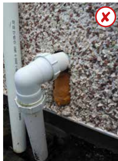
Figure 35: Unsealed pipe penetration
