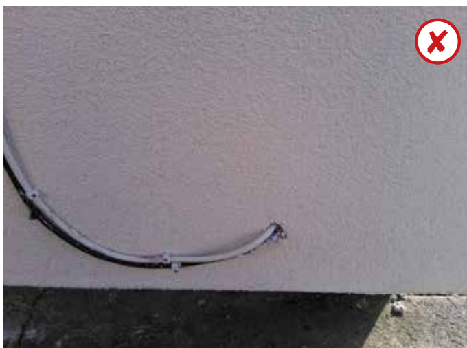
Figure 36: Unsealed wire penetration
