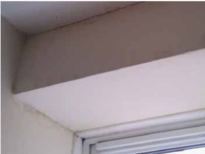
Figure 50: Damp in the kitchen
