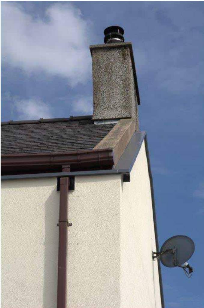
Figure 33: Roof of the building not extended to protect the insulation
