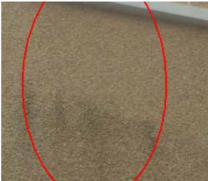
Figure 45: Staining by lack of capillary drip
